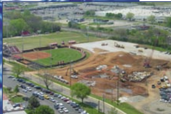
Western Kentucky University - Vortechs installation
